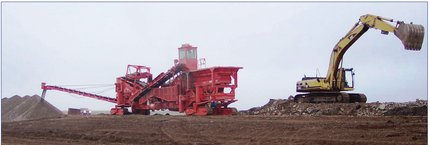
Figure 4. Paradigm in-place concrete recycling equipment in operation in Oklahoma (photo courtesy of Duit Construction)
